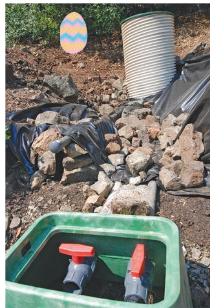
Spring site with county-approved spring box piped to a control station. Notice the start of the back fill using pond grade plastic. Very important to protect the ground around the site.
