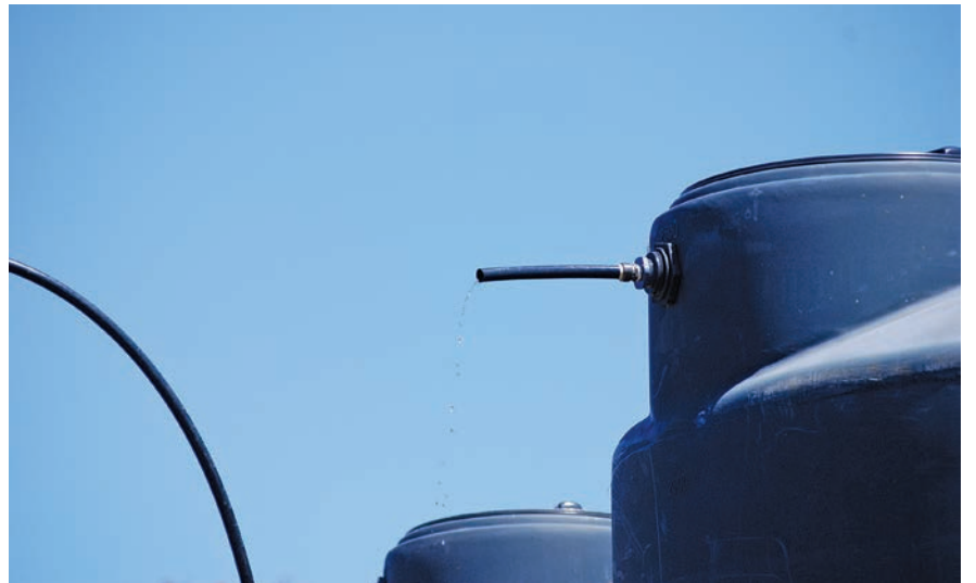
The final stage of the water’s journey is the storage tanks. The arching ¾-inch Schedule 80 pipe is the end of the delivery line. These tanks are filled from the ground up, and the water dripping out is simply overflow.
