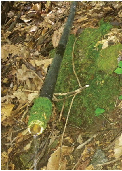
Broken spring box still putting out near 0.3 GPM. Check the moss. The plastic pipe dates its use. The cement spring box in the corner also dates itself. For that, I am guessing near the turn of the last century.
