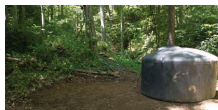
The tank site is prepped, making it level for the rocks and with enough room for the pipes.
