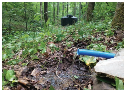
Just 25 feet away from the tank site, this is the end of a 500-foot travel from the spring box.
