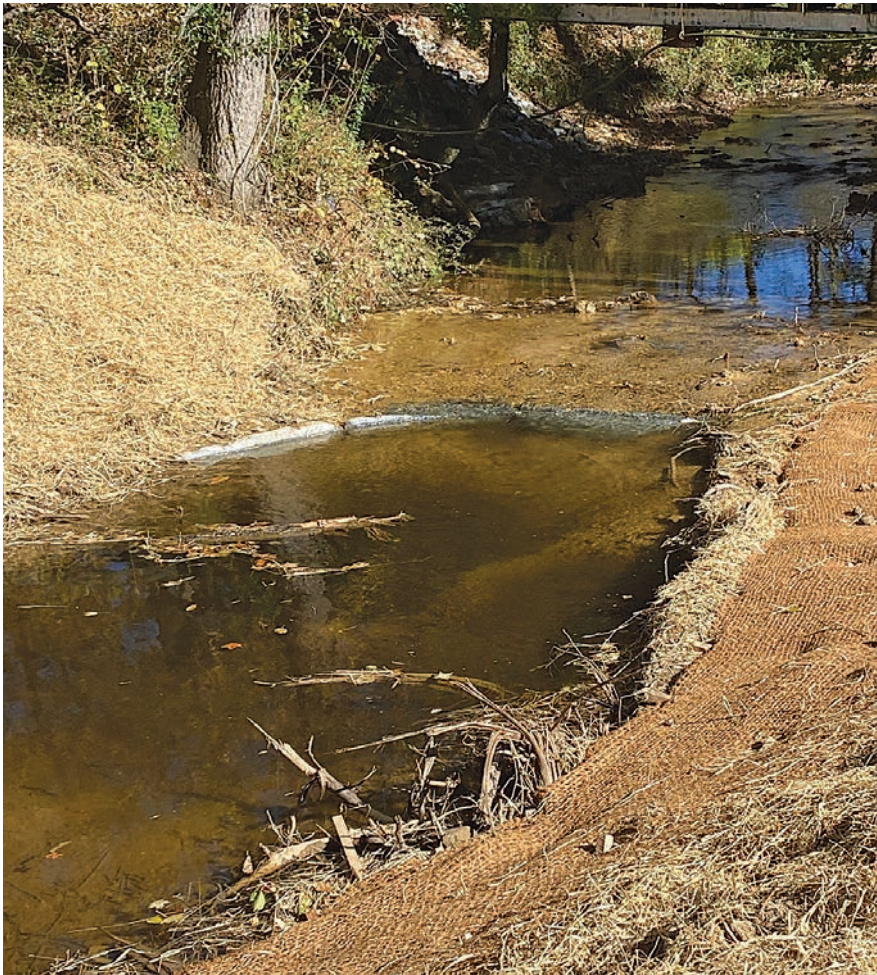
In this log-and-rock vane design, the log (right shore) protects the bottom of the sloped bank while the curve of large rock slabs across the stream directs flow to create a deep pool in the center.
