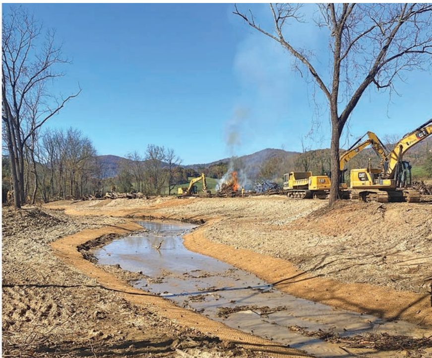
The new, curving channel and more gently sloping banks were created by the heavy equipment in the background. Although many trees were removed, the new plantings will all be native trees and shrubs of much better diversity than the former vegetation.
